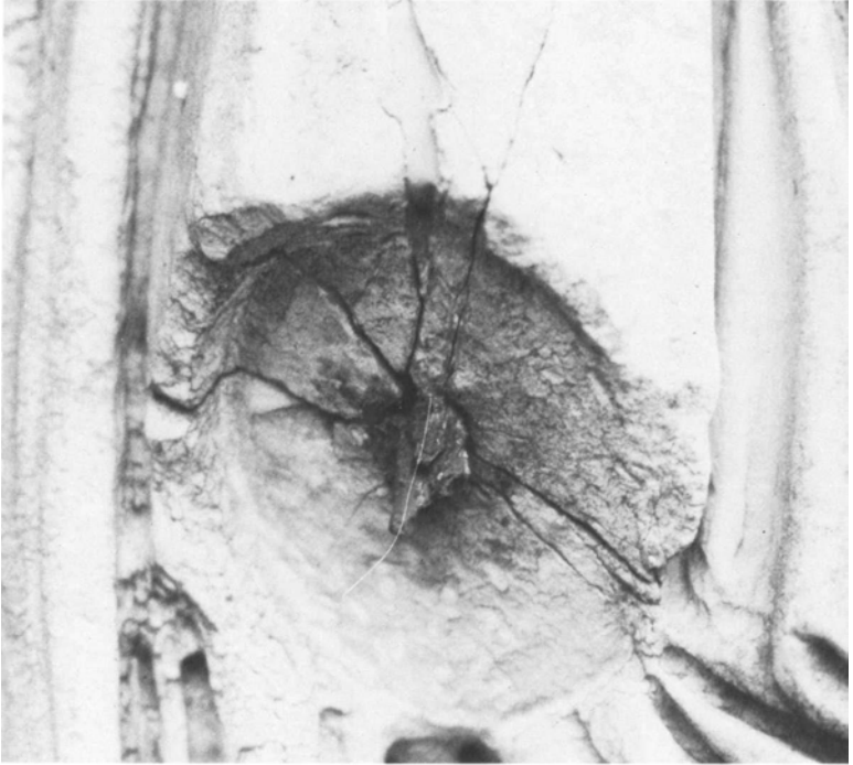
Fractures caused by the inclusion of iron pins
