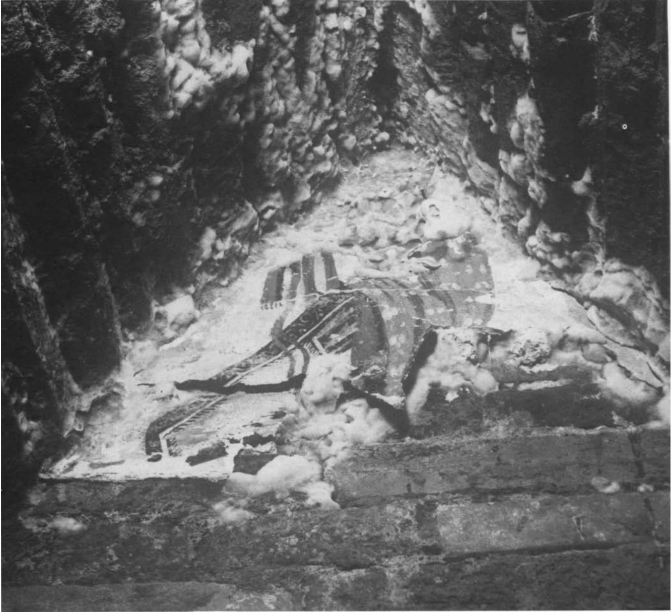
3 Ceiling and south pediment: the funghi bloom.
